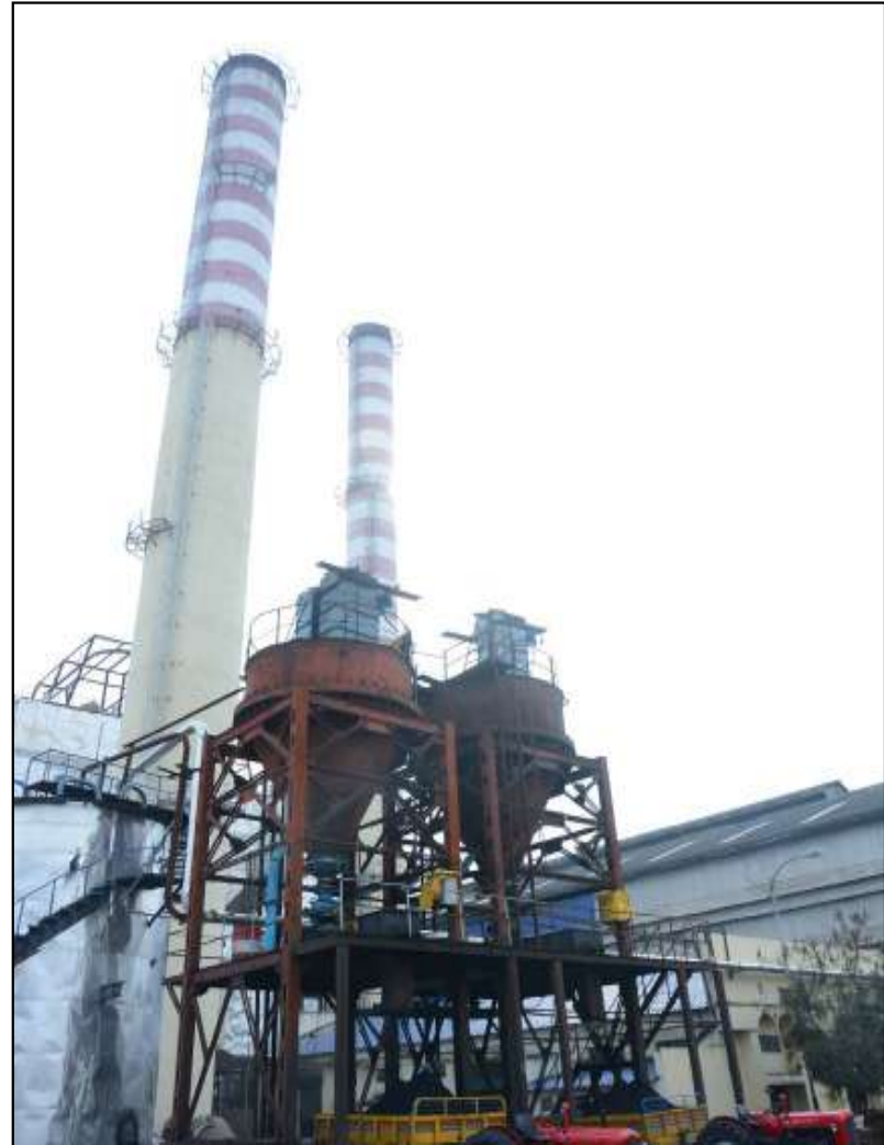
Boiler Ash Handling System
